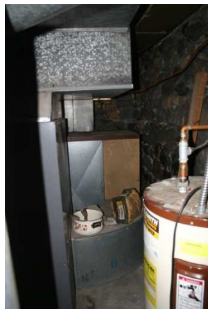
ERUM, Sept. 11, FURNACE ROOM
