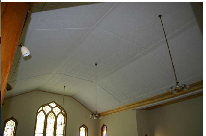
ERUM, Sept 2011, Ceiling with lighting
